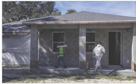
People work on the insulation of a home under construction in St. Petersburg on Monday. Building costs have skyrocketed.
